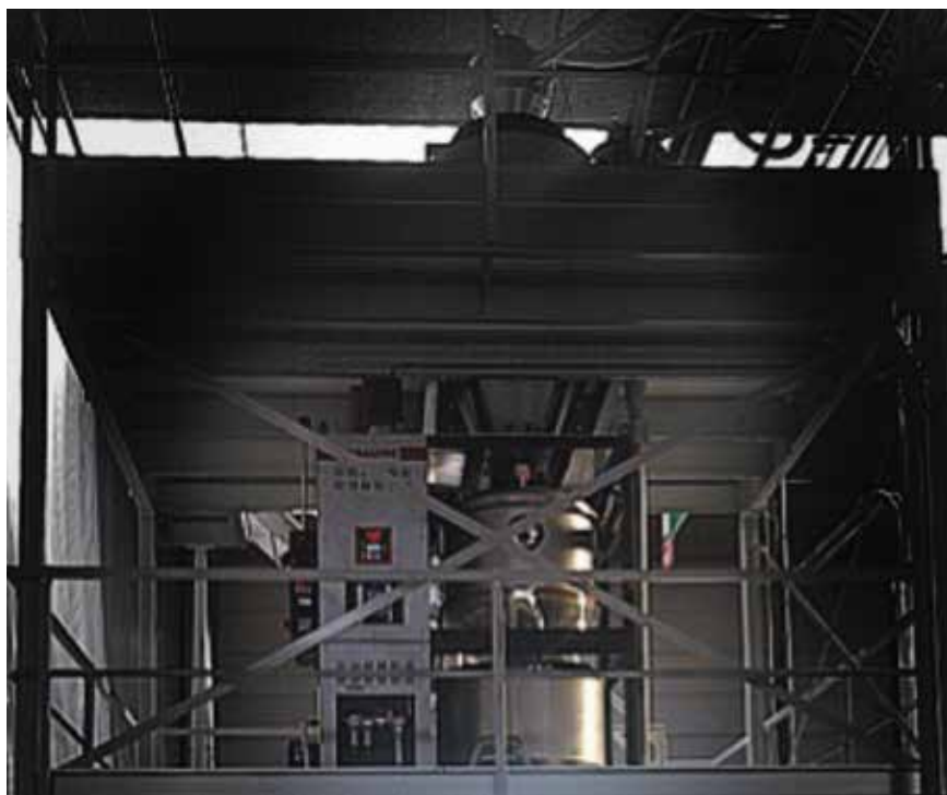
VBD-1000 installed on mezzanine
